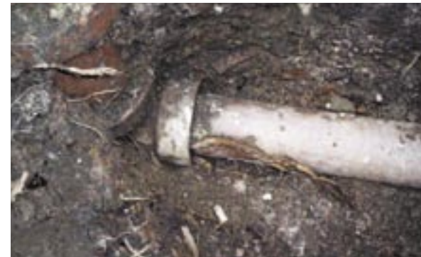
ROOTS ENTER THROUGH CRACKS AND JOINTS BEFORE GROWING THICKER AND BREAKING THE PIPE OPEN
