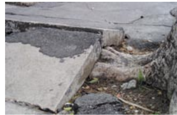
TREE ROOTS ARE VERY POWERFUL AND WILL EASILY DAMAGE SEWER PIPES, BRICKWALLS AND FOUNDATIONS
