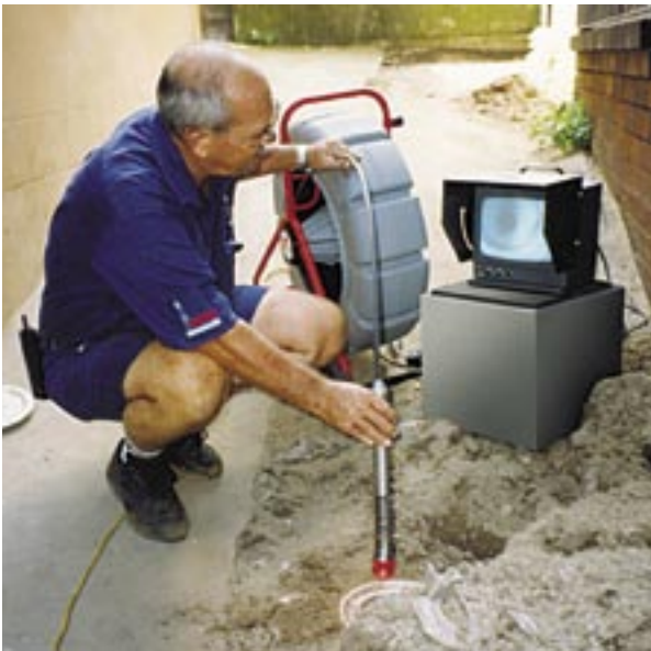
Your Mr Washer Plumber will carry out a Camera Inspection of the pipe to ensure Vaporooter II is the best way to solve your problems.
