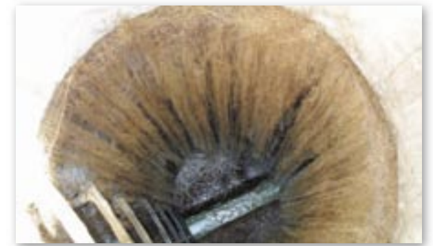
A VEIL OF ROOTS IN A MANHOLE BEFORE TREATMENT WITH VAPOROOTER
